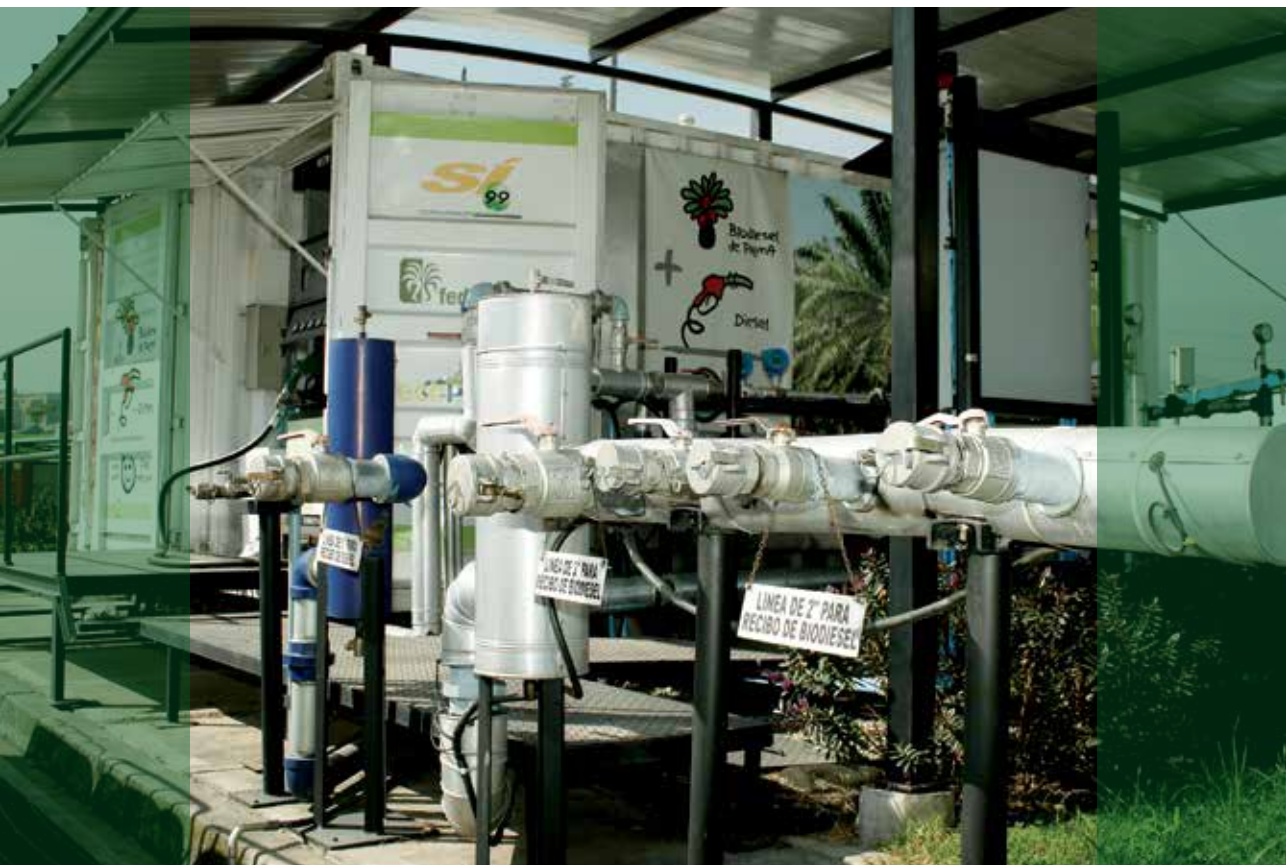
Receiving lines for oil palm biodiesel at the blending station. Photography: Gutiérrez, R. y Holguín, J. L. (2008).
